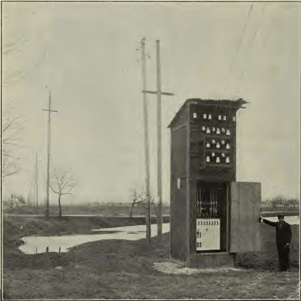
HORDORF SUB-STATION, CROTTORF AGRICULTURAL ELECTRIC INSTALLATION.
